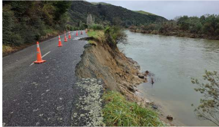
^ Damage to the Westbank Road below the Pearse confluence. Photo: Rhys Barrier.
