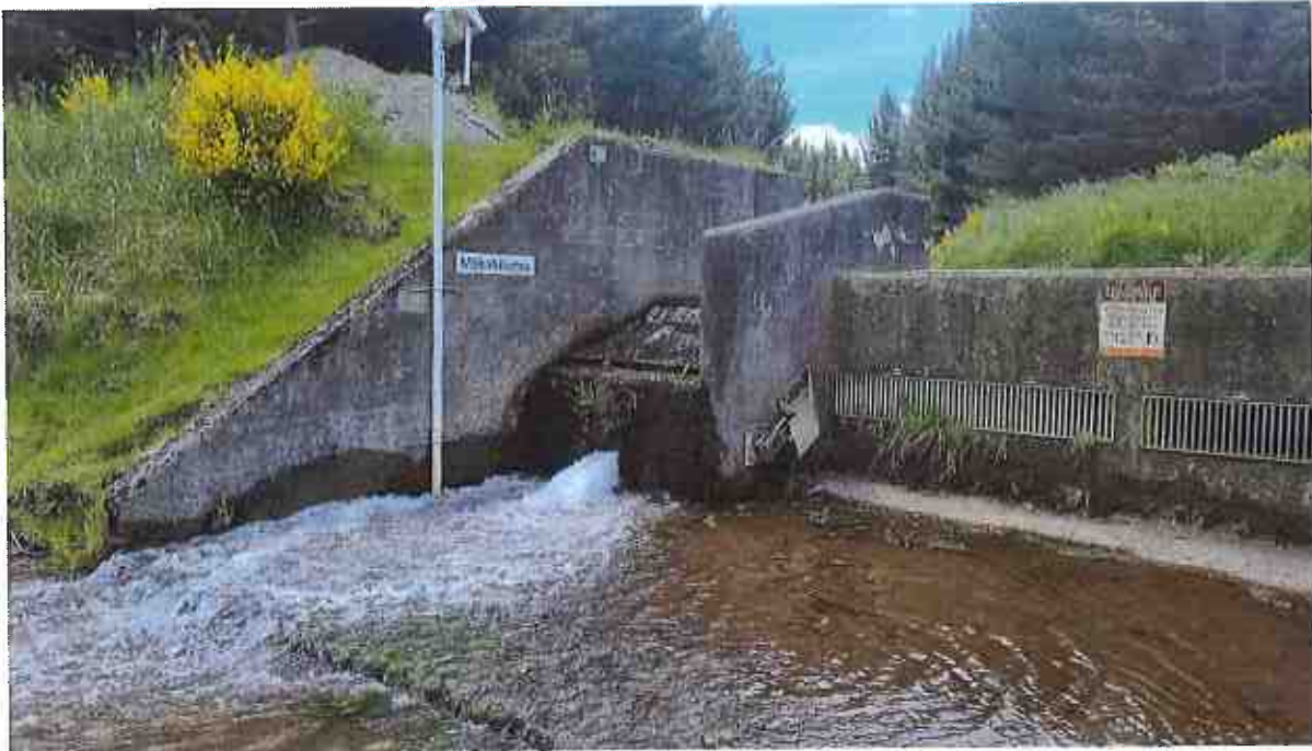
Photo 1. Tongariro HEPS Eastern Diversion structure on Mākahikatoa Stream showing downstream residual flow, 4 th December 2024.
