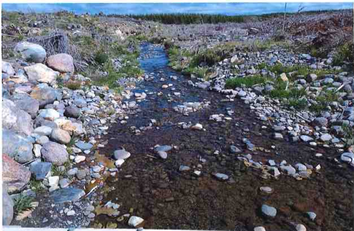
Photo 14: Tokiāhuru Stream tributary Link Road box culvert, downstream site (Site 8), 5 th December 2024.
