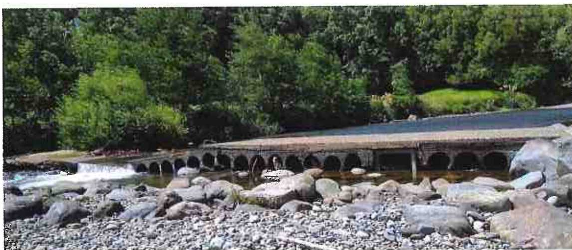
Photo 27. Disused concrete ford in the Manganui River mainstem just upstream from the Waipuku Stream confluence.
