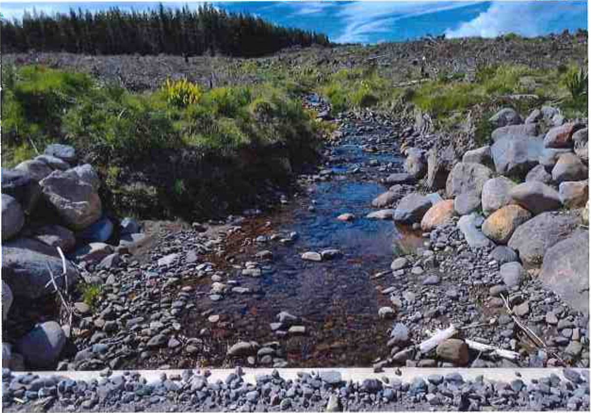
Photo 13: Tokiāhuru Stream tributary Link Road box culvert, upstream site (Site 8), 5 th December 2024.
